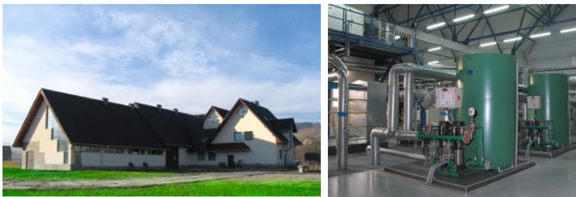
Figure 3.1 The peak load boiler house
